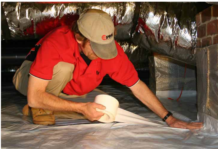
Photo courtesy Crawlspace Care Technologies, Inc.
