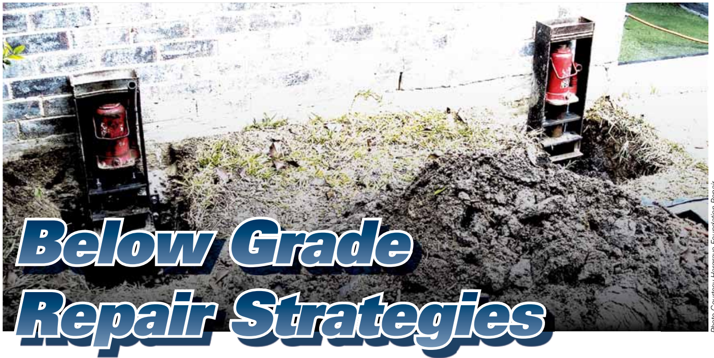
Photo Courtesy Hargrave Foundation Repair
