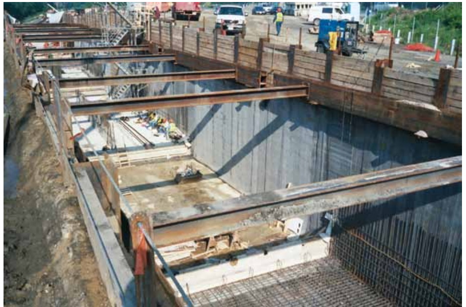
The Washington D.C. Blue Line tunnel is an excellent example of cut-and-cover construction. More than 1.3 million sq. ft. of Voltex DS, a bentonite sheet membrane, was applied to the walls and floor, the top was sealed with rubberized asphalt.
