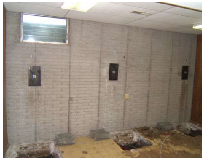
Wall anchors require significant excavation. Metal plates on the interior (at right) keep the wall from bowing further.
