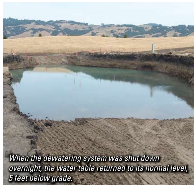
Temporary pumps removed up to 400,000 gallons of water a day to allow basement excavation to proceed.
